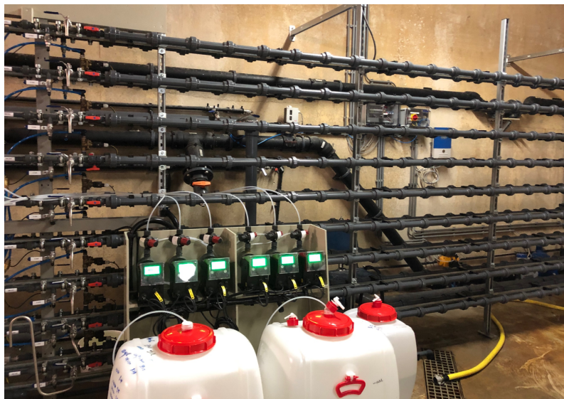
Figure 3.1 Pilot system on site
