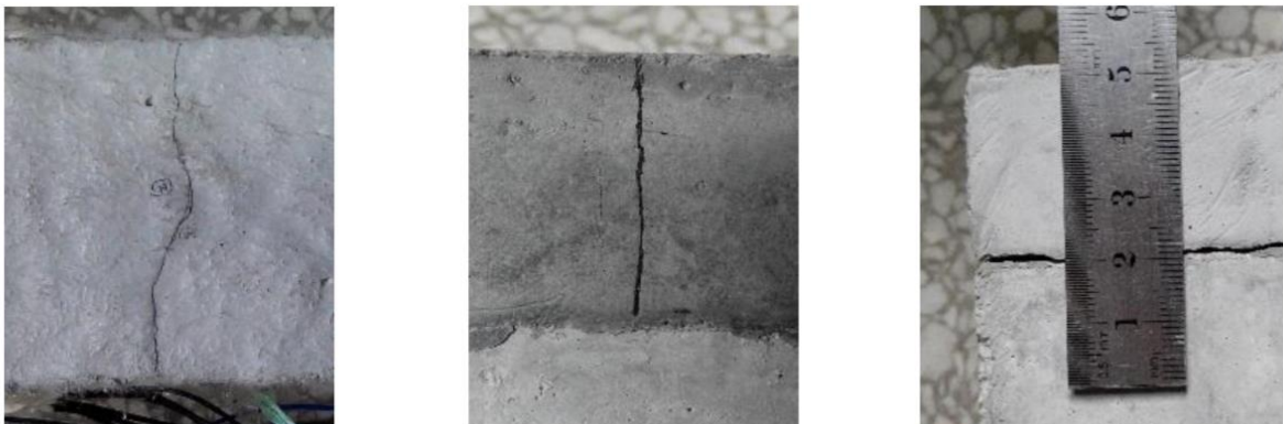
Figure 4. Failure modes of SHCC-repaired beams due to shrinkage [29].
