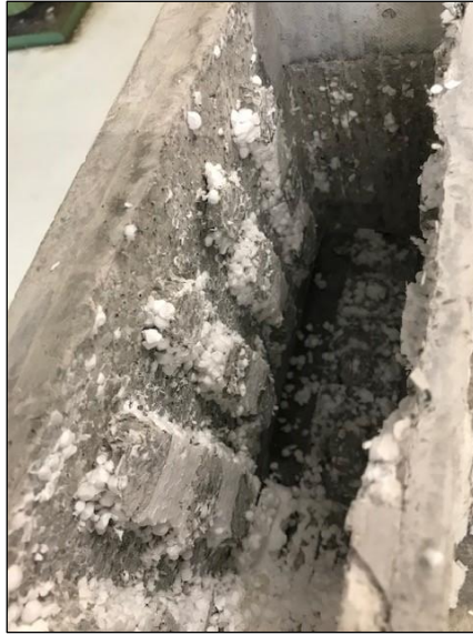
Figure B.3. Shear keys on the surface of the U-shaped SHCC formwork after removing Styrofoam.
