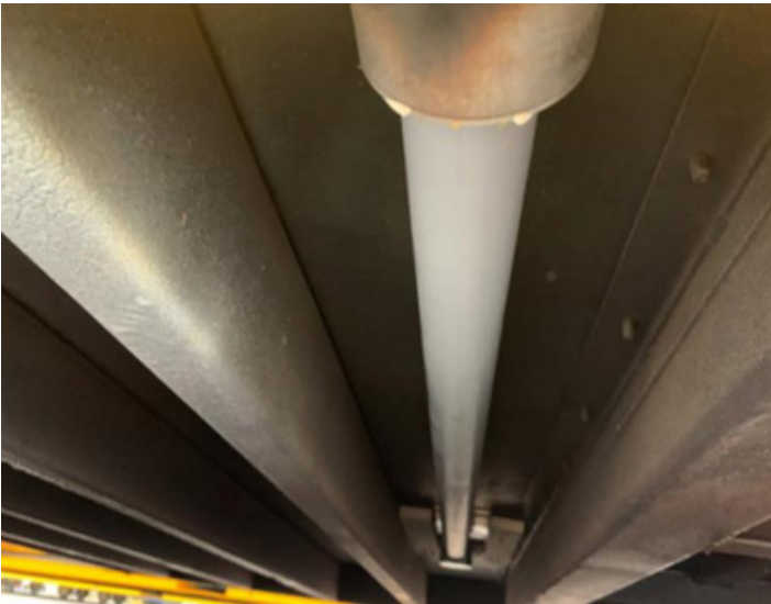
Figure 135: Drains underneath container
