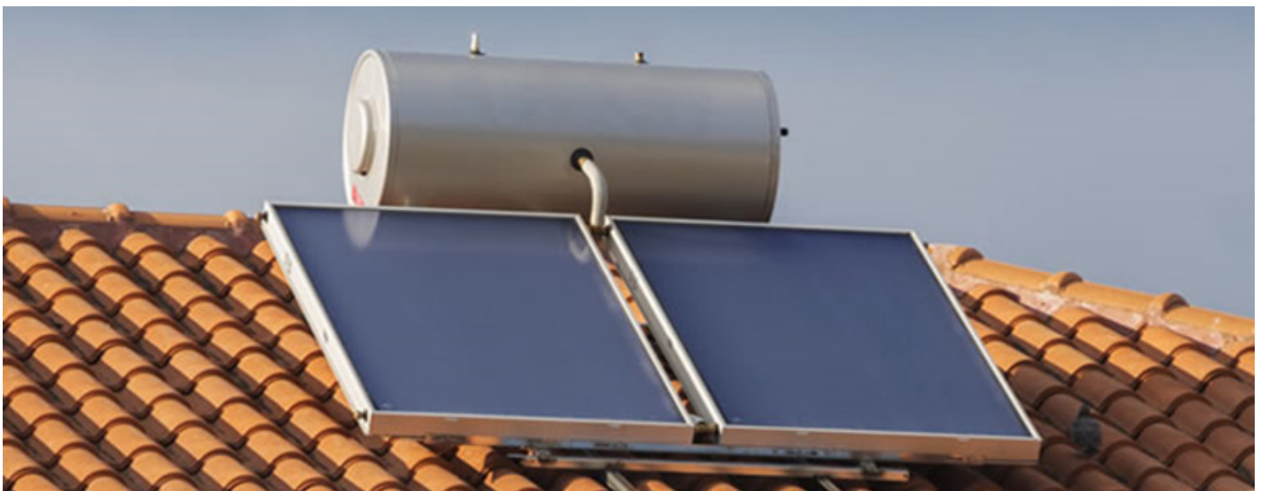
Figure 1: Solar heating panels
