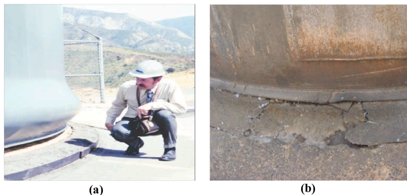
Fig. 3. Elephant-foot buckling and cracked foundation of steel tanks, (a) Elephant-foot buckling of a tank wall (courtesy of University of California at Berkeley) [38]; (b) Cracked foundation of the tank during the Silakhor Earthquake of 2006 in Iran [34].
