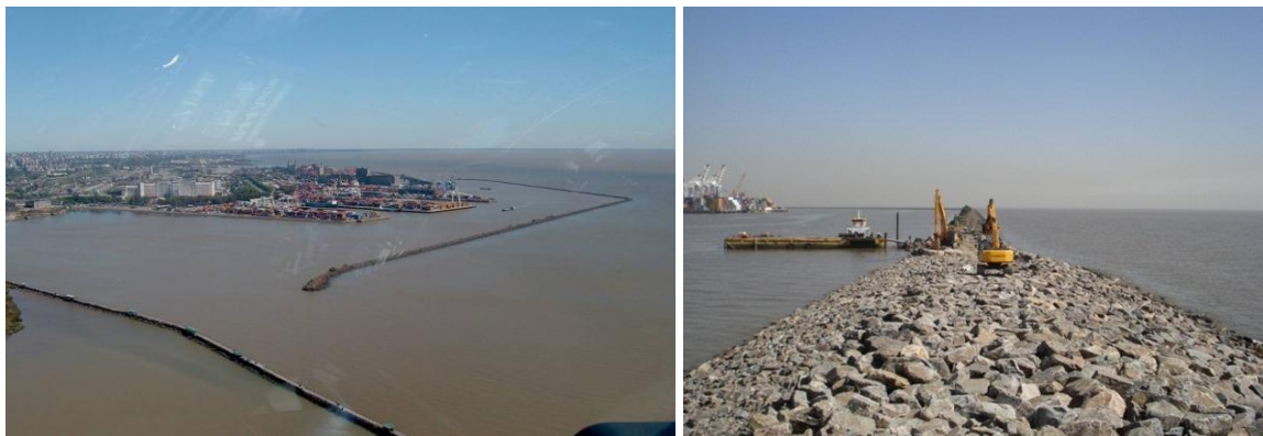
Figure 6-3. Improvement of an estuarine rubble mound breakwater at Port of Buenos Aires, Argentina, 2012
