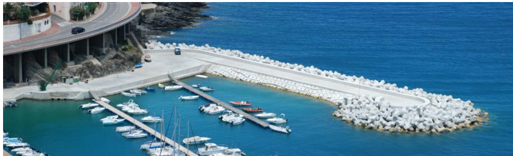
Figure 6-13. Breakwater reconstruction, Cerbere, France (maximum unit size 9m 3 and water depth 10m), 2010
