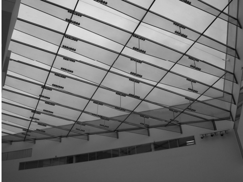
Fig. 1.26 Atrium roof of the Wolfson Building, architectural design by Reich and Hall, glass design by Arup, 2002, Glasgow, UK.
