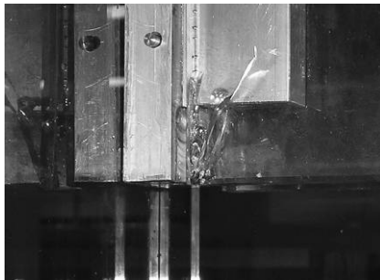
Fig. A.22 Damage in this purlin did not induce complete element failure because annealed glass was used.
