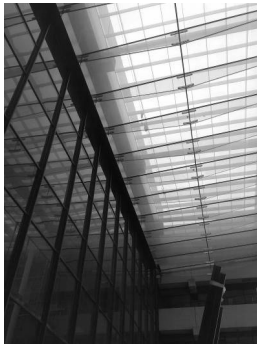
Fig. 5.8a Allied Irish Bank (AIB), Dublin, Ireland. Span: 8 m. 2 Sections of 3x12 mm heat strengthened glass. PVB laminated. 2007. Façade design: Arup, London, UK. Structural glass engineer: Gartner Steel and Glass, 11 Würzburg, Germany.
