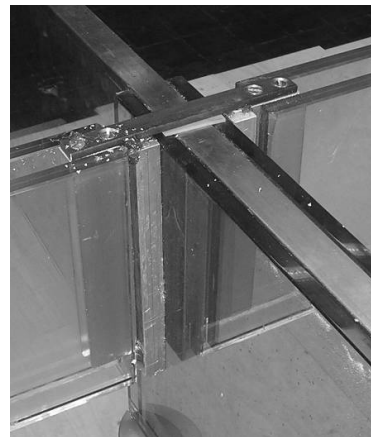
Fig. 2.10 A steel bridge over the main beam serves as a back-up for the adhesive bond between the aluminium joint component and the glass.
