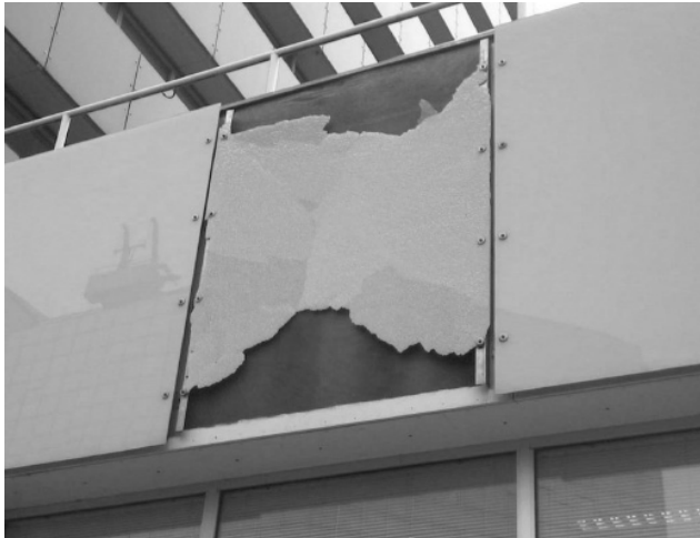
Fig. 5.30 Thermally toughened glass does not always break into small humps immediately upon failure.
