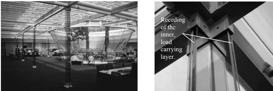
Fig. 5.5a, b Structural glass column, town hall of Saint-Germain-en-Laye, France, 1994. Overview (left) and detail (right), with the receding inner layer visible. In this design, only the inner layer is load carrying. Architect: Brunet et Saunier, Structural Engineer: OTH/Alto – M. Malinowski.
