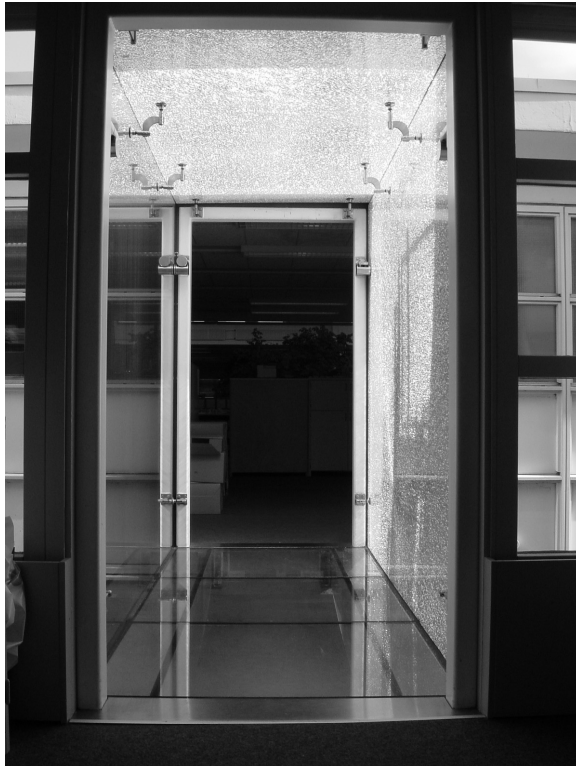
Fig. 5.31 Glass bridge in Rotterdam after treatment by vandals: the inner layers of the roof and wall panels proved to be sufficiently protected not to break and to keep carrying loads.
