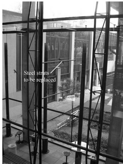
Fig. A.38 The Faculty of Architecture has been extended with a smoking room; essentially a glass box added to the existing glass façade (picture taken from inside the Faculty building). The two steel struts which are to be replaced are visible in the centre of the picture.
