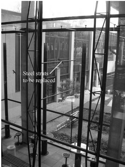
Fig. 2.18 The Faculty of Architecture has been extended with a smoking room; essentially a glass box added to the existing glass façade (picture taken from inside the Faculty building). The two steel struts which are to be replaced are visible in the centre of the picture.
