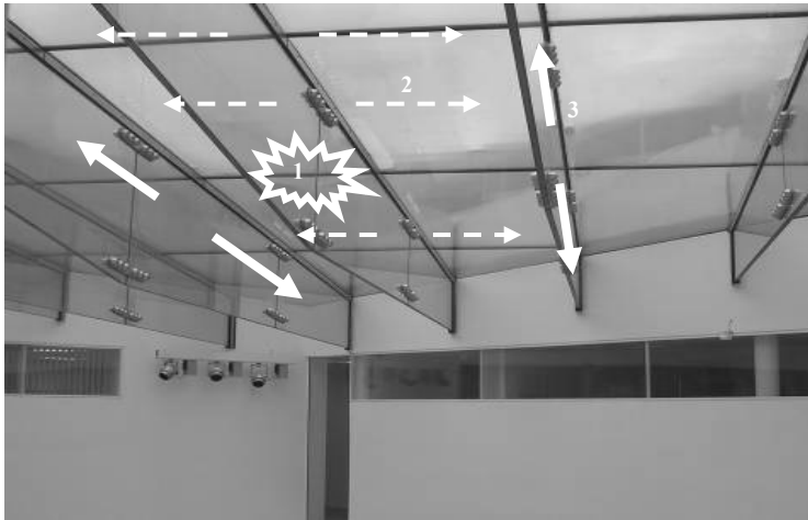
Fig. 8.26 Alternative load path in the Wolfson Building glass roof, Glasgow, UK. In case one beam loses all load transfer capacity (1), loads can be redistributed to the adjacent beams (3) through catenary action (perpendicular to the beam length axis) in the roof panels (2).
