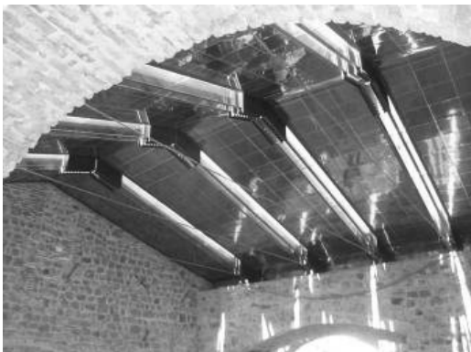
Fig. 5.15a Loggia dei Vicari, Arquà Petrarca (PA), Italy. Span: 11 m. 2 Sections. 4 layers, annealed glass. PVB laminated. Carbon fibre reinforcement strip. ~ 2004. Structural glass engineer: Vetrostrutturale, Brescia, Italy.
