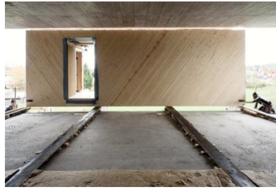
Figure 5.4. Installation of the modules using wheels running on rails (Sobek et al., 2018).
