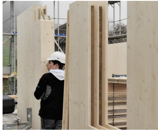
Figure 5.14. Assembly of ECO Solar Houses in Saint Margrethen using the ECOCELL system (ECOCELL, n.d.).
