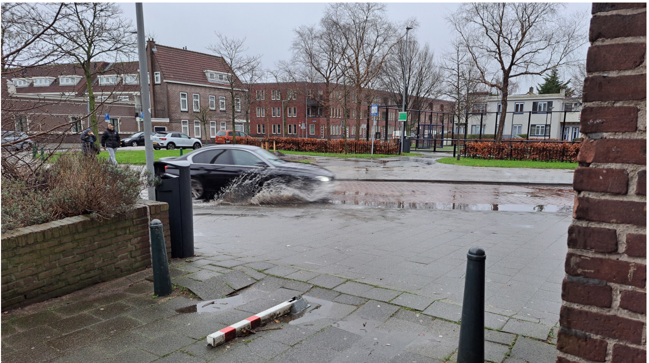
Figure 4.1: Site photo with damaged sidewalk, speeding cars, and in the background the large building blocks
