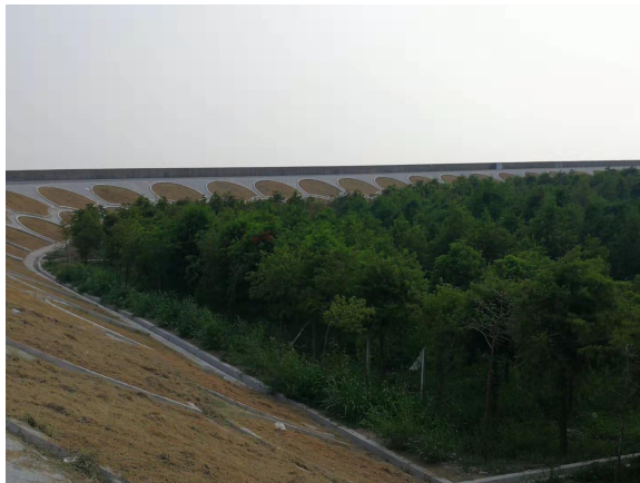
(b) Yellow grasses on the slope at location A
