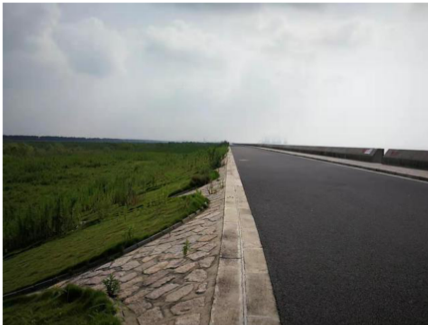
Fig. 4.3.: Typical inner slope of sea dikes in Shanghai, taken during the field work in Shanghai
