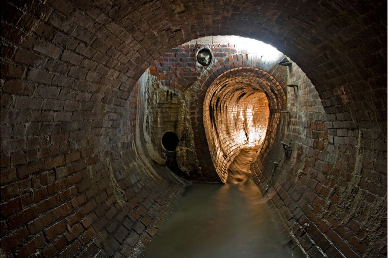
Midway Combined Sewer
