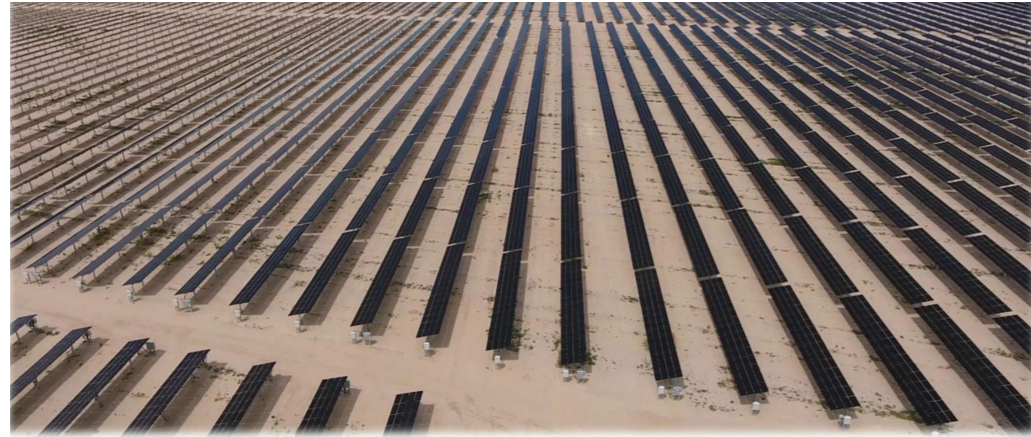
Photo Credit: East Pecos Solar 120MW AC , Texas, Southern Power
