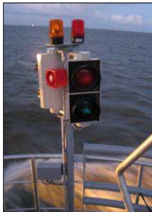
Figure 5.10 Alarm tree on transfer deck
