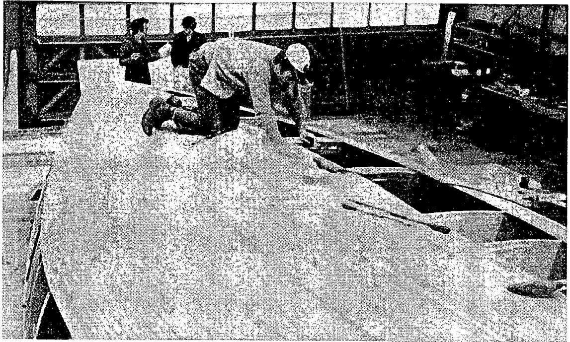
Figure 5. Strip planking that is neither tapered nor beveled (to save time) is temporarily fastened to the mold frames until the bonding adhesive between the plank edges reaches a cure. The planks are also bonded to any permanent members in the set-up.
