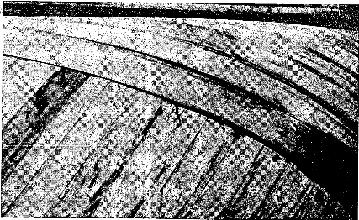
Figure 3. The \frac{1}{8} inch thick veneers were held in place with staples until a resin cure could take place. After the first two layers were bounded, the alloy staples were left in place on subsequent layers to save time.
