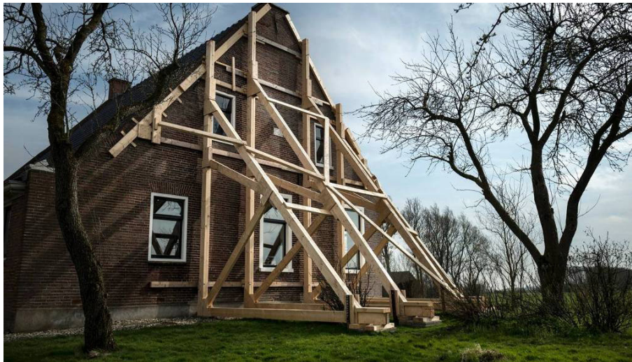
Figure 15: Pictures of a farm in Groningen that is scaffolded against seismic actions (Groningen, 2015)
