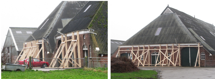
Figure 12: Pictures of a farm in Groningen that is scaffolded against seismic actions (Groningen, 2015)
