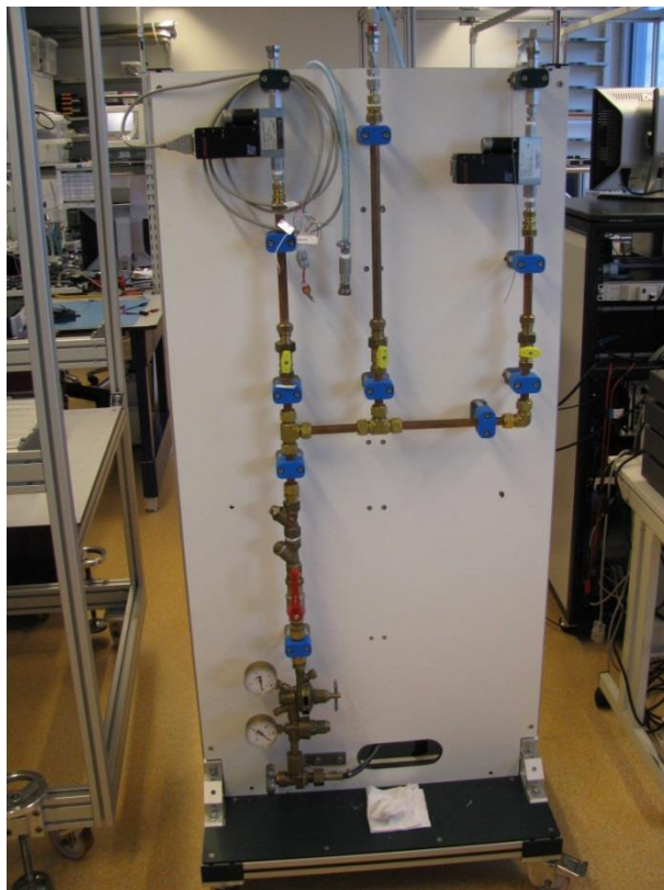
Figure 71: Nitrogen Tank and Pressure Regulator
