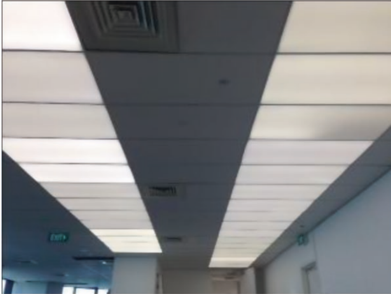
Fig. 7.16 Example of color maintenance drift for an indoor installation
