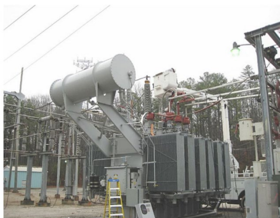
Fig. 1. TDSF monitoring in a 230 kV/20 kV, 60 MVA distribution substation transformer.
