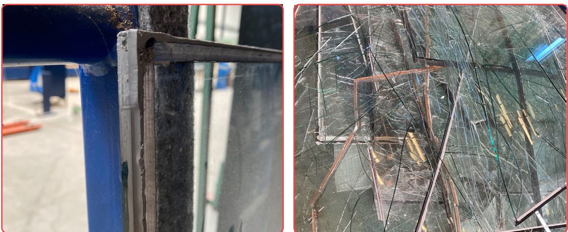
Figure 3.73. Glass separation, material loss due sealing compound (left). Glass sent to landfill (right). (Images by Author).
