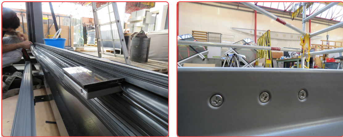
Figure 3.74. (left) Triodos Bank Mockup: Disassembly of Gaskets. (right) Screws used in window-frame assembly. (Octatube, 2018).
