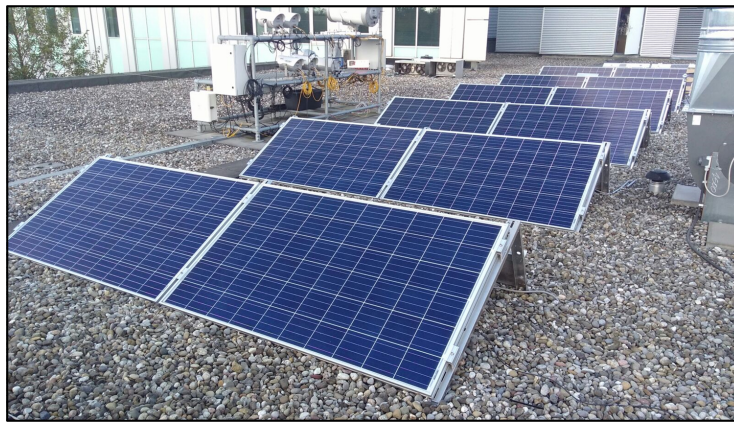
Figure 2.3: Rooftop PV setup for soiling experiment.
