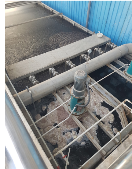
FIGURE 30. Water treatment (H. Teeuwen)
