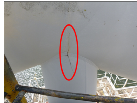
Figure 15: Present found cracks
