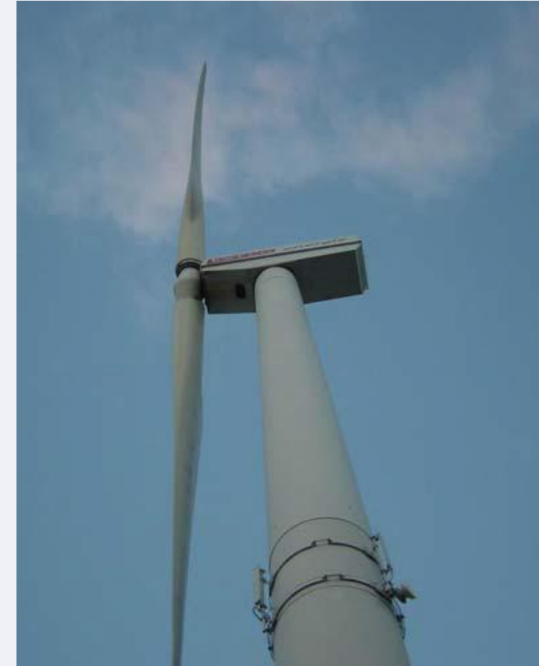
Figure 2: Slip joint connection on a wind turbine at Scheveningen in the Netherlands [1].
