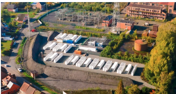
Figure 2.2.1: 200 MWh BEss FCR facility in Belgium. Image: Corsica Sole
