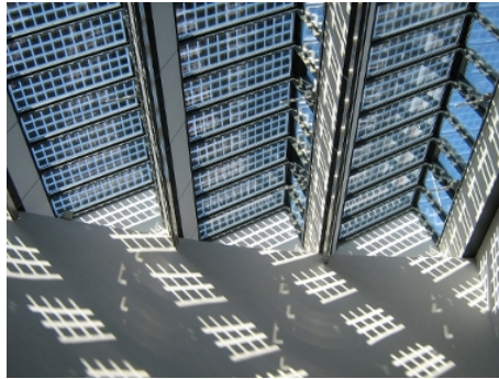
Figure 4.41: A view of the saw-tooth roof BIPV system from the interior of the Fraunhofer ISE main building. The shadow pattern on the interior walls caused by the BIPV system is clearly visible. For lower solar altitude angles, the shadow pattern of one module row can be transmitted through the north-facing windows of the sawtooth structure onto the modules of the next row.
