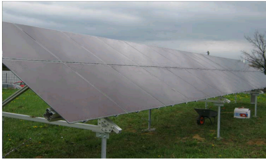
Figure 4.50: The PV system in Mochau, consisting of 30 PV modules based on amorphous silicon. The PV modules were manufactured by the company Signet Solar and are arranged in two rows of 15 PV modules each. Source: SunStrom
