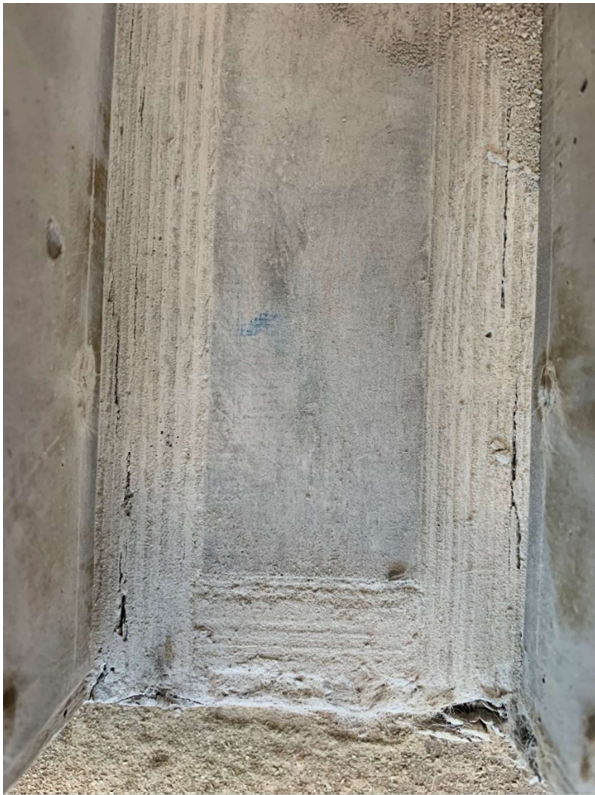
Appendix figure 64: longitudinal cracks as a result of excessive hammering during demoulding
