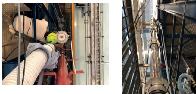
Figure D.2: Left, a top view picture where the set-up is under construction. Right, a side view of the complete set-up.
