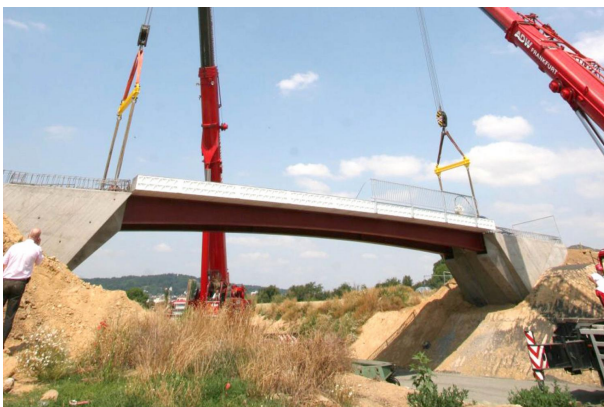
Figure 2: Friedberg Bridge, Germany. This bridge has a width of 5 m and a span of 27 m. A multi-cell platform deck made of FRP profiles rests on two steel beams. The deck and the beams were glued in-situ to each other [10].
