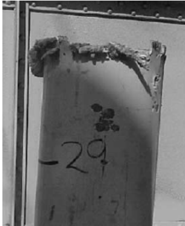
Figure 24: Damage after driving on pile head [16]
