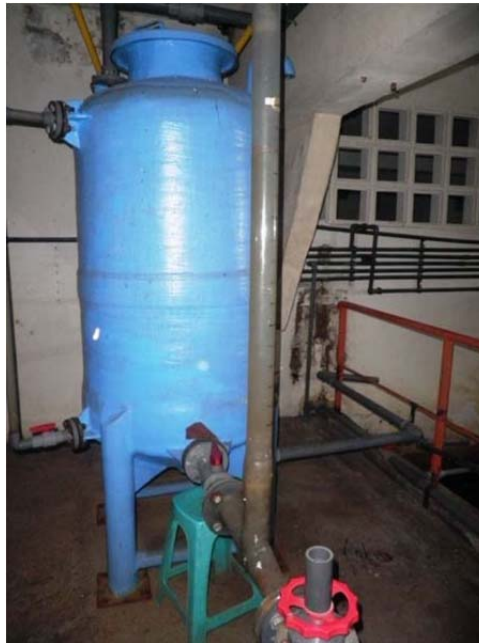
Figure 3. 3 PAC dosing tank
