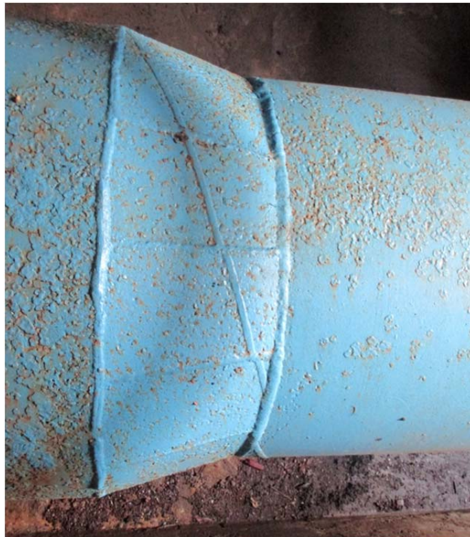
Figure 2. 7 Location at OVS1 Pipa Baru where the butterfly valve was removed and pipeline was welded back together
