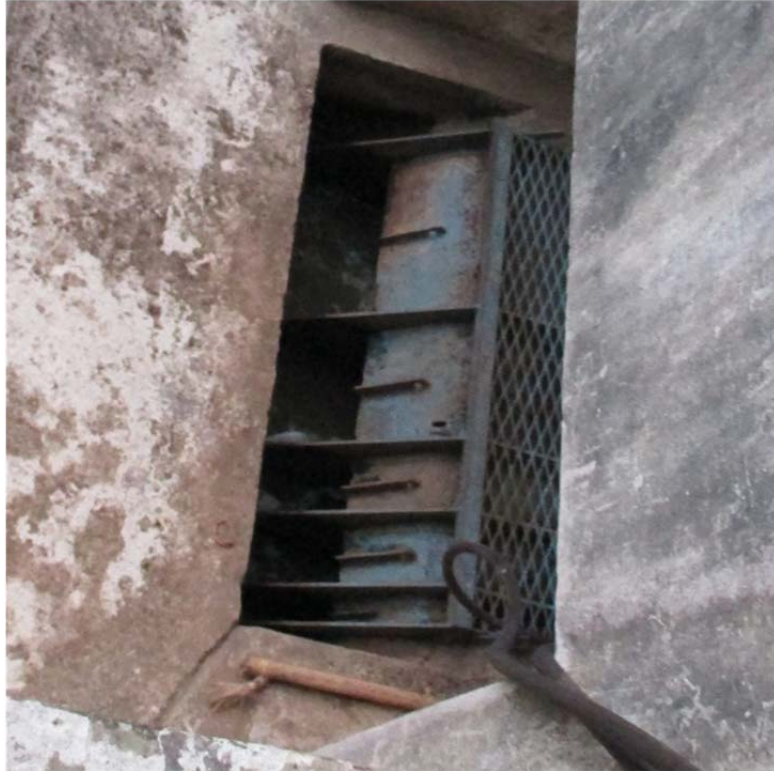
Figure 2. 5 Discharge measurement in Hydroelectric power plant upstream of PDAM Cikalong
