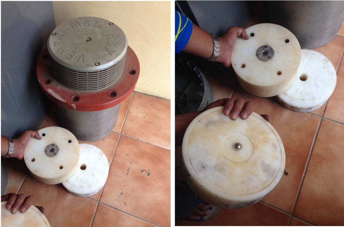
Figure 2.9 New type of air valves along Pipa Baru
