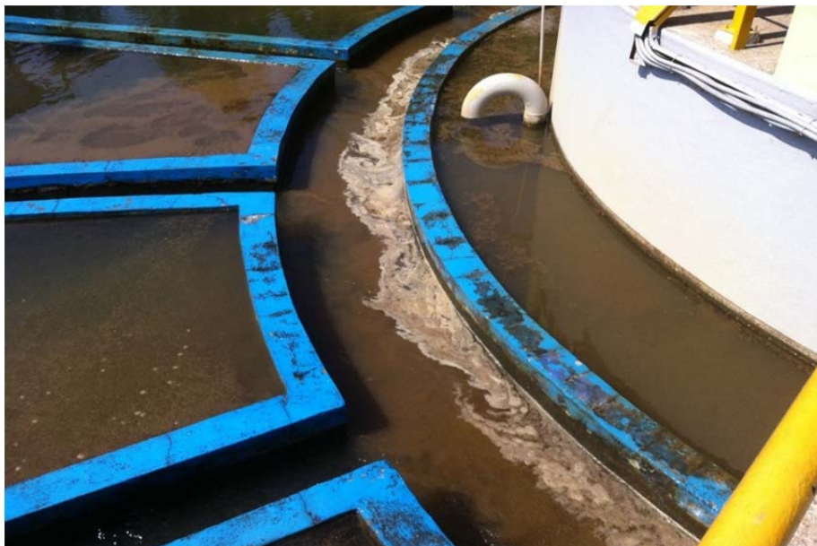
Figure 3. 25 Effluent contaminated with sludge after the cleaning procedure
