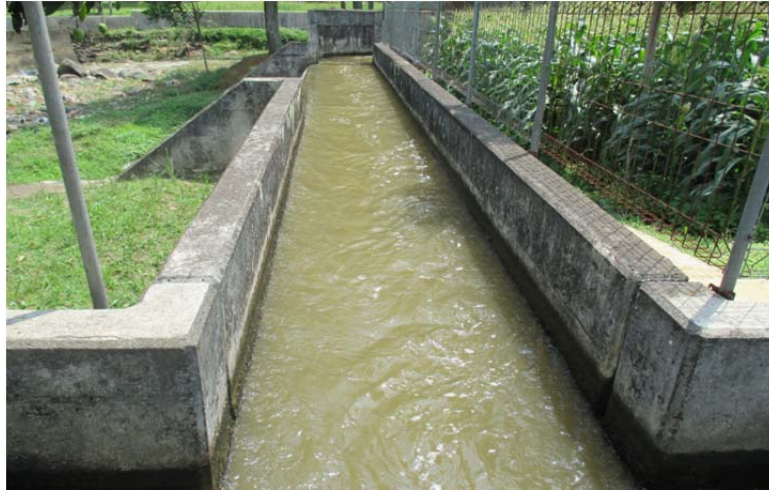
Figure 1. 8 Open Channel from PLTA Cikalong Discharge
