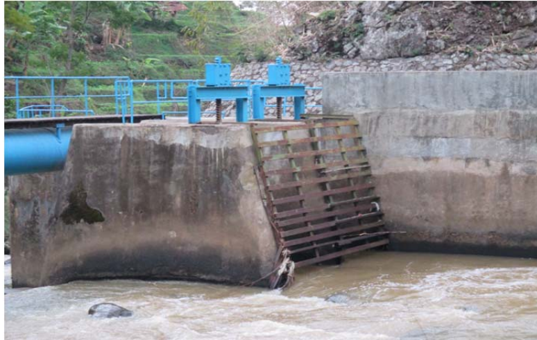
Figure 1. 10 Pipe Bridge Connection and Collecting Pond
