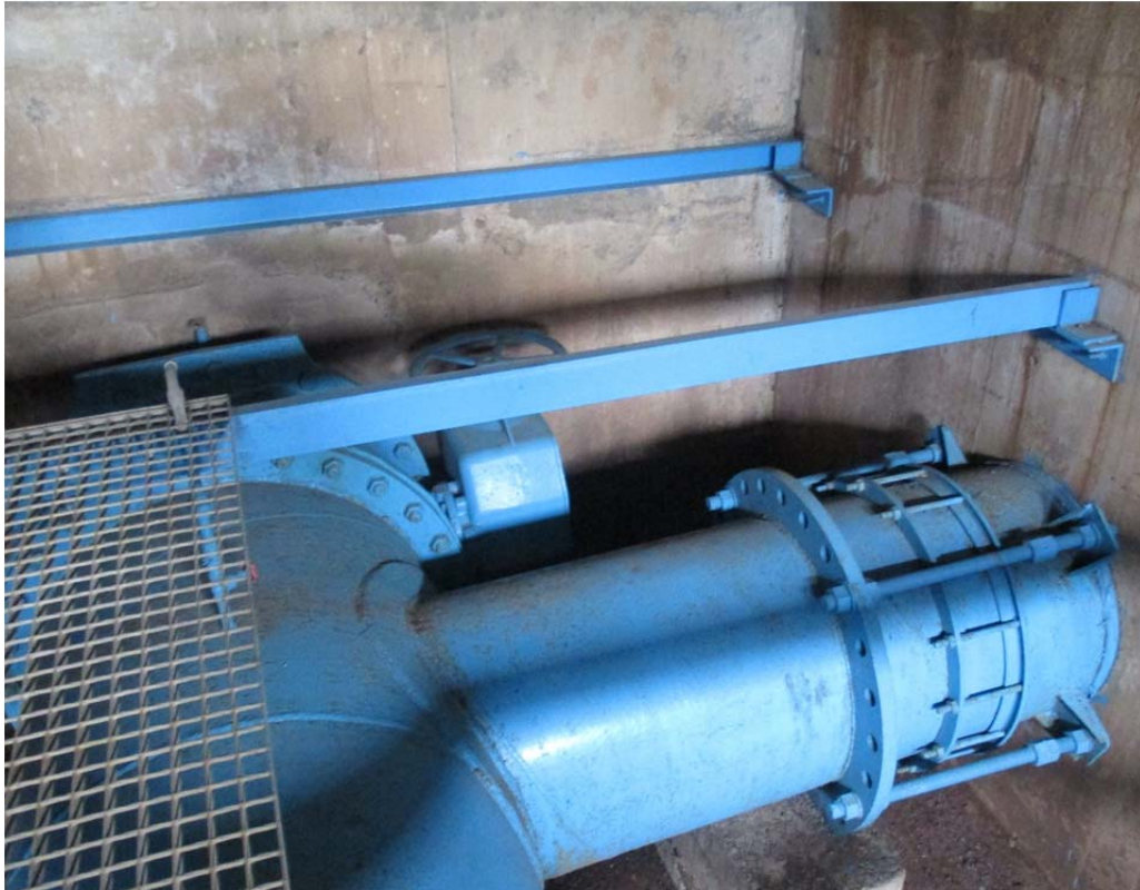
Figure 2. 8 Interconnection between Pipa Baru and Pipa Lama at OVS1, and butterfly valve after the interconnection
