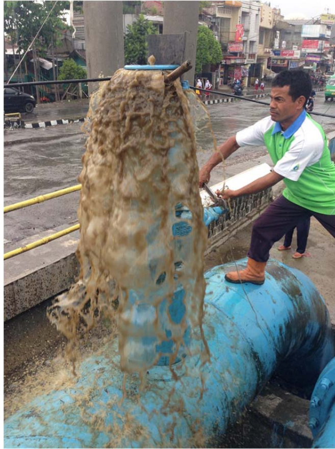
Figure 2. 10 Air valve maintenance
