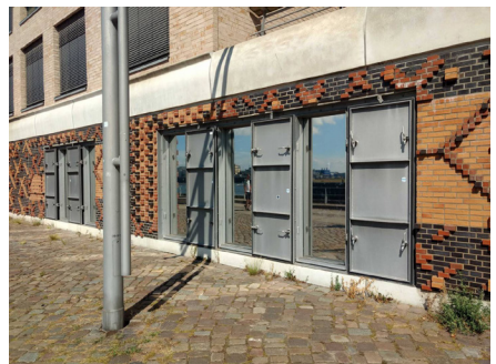
Figure 37: Watertight shutters (KCAP, 2020)
