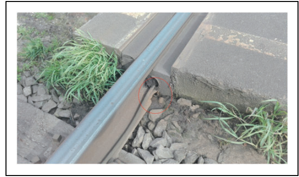
Figure 3. Reduced profiles in rail foot caused by corrosion (ProRail inspection photo).
