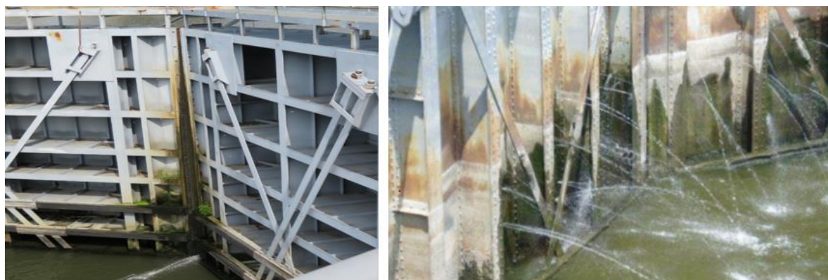
Figure 1: Two lock gates at exceeded life time and in need of maintenance and renovation: Left: seepage through centre seal between mitre gate doors. Right: corrosion leading to overall seepage (Buildiww, 2018)
