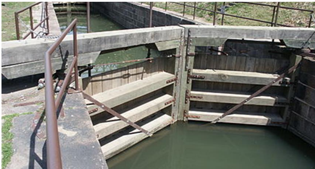
Figure 77: Wooden Mitre Gate
