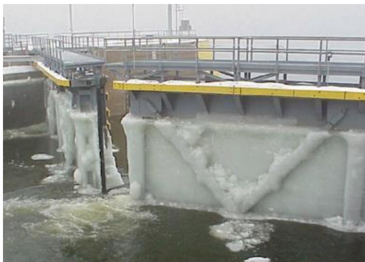
Figure 33: Adherent ice on mitre gates (Johnson, 2017)
