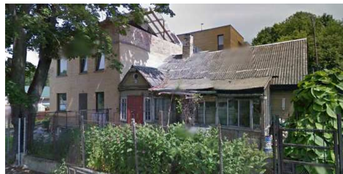
FIGURE 46. HALF OF THE HOUSE BEING REBUILD. NAUJININKAI, VILNIUS. STRUCTURE OF OLD WOODEN LITHUANIAN HOUSES ALLOWS PARTIAL DEMOLITION IF IT IS NOT DEMOLISHED LENGTHWISE. SOURCE: GOOGLE STREET VIEW.
