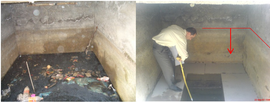
Figure 9: Sewage filled outlet of Qanat, before and a couple of days after revitalization.
