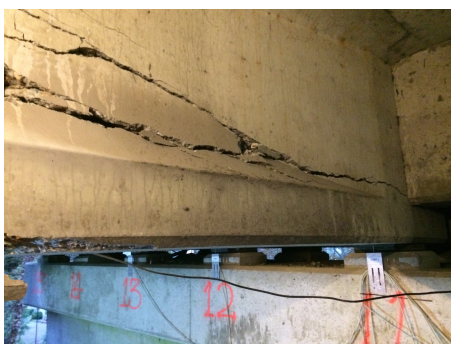
(a) Shear cracks towards end support
