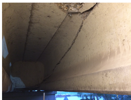
(b) Shear crack towards intermediate cross-beam
