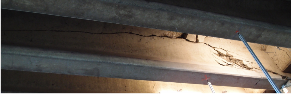
Figure 6.34: Shear failure T-beam test 2 (intermediate cross-beam on the left side, end support on the right side)
