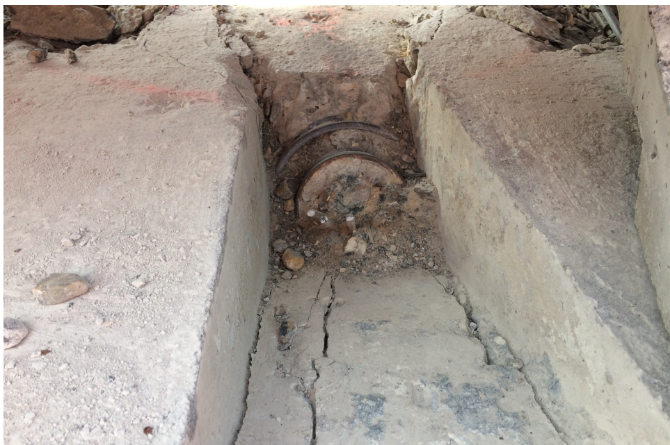
Figure 6.40: Broken out unreinforced concrete filling at anchorage of tendon 7 in tests 4-6 (see Chapter 5 Figure 5.6). View towards span, the load position is just visible at the top side of the photo
