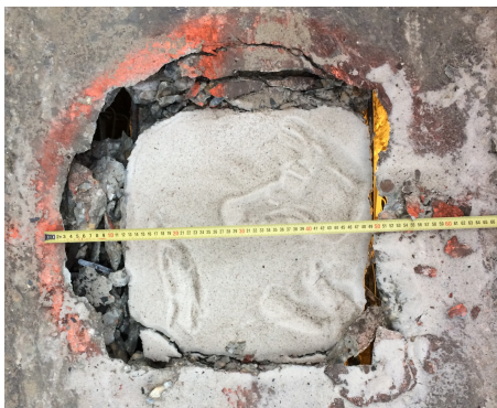
(a) Punching failure top side (measurements in cm)
