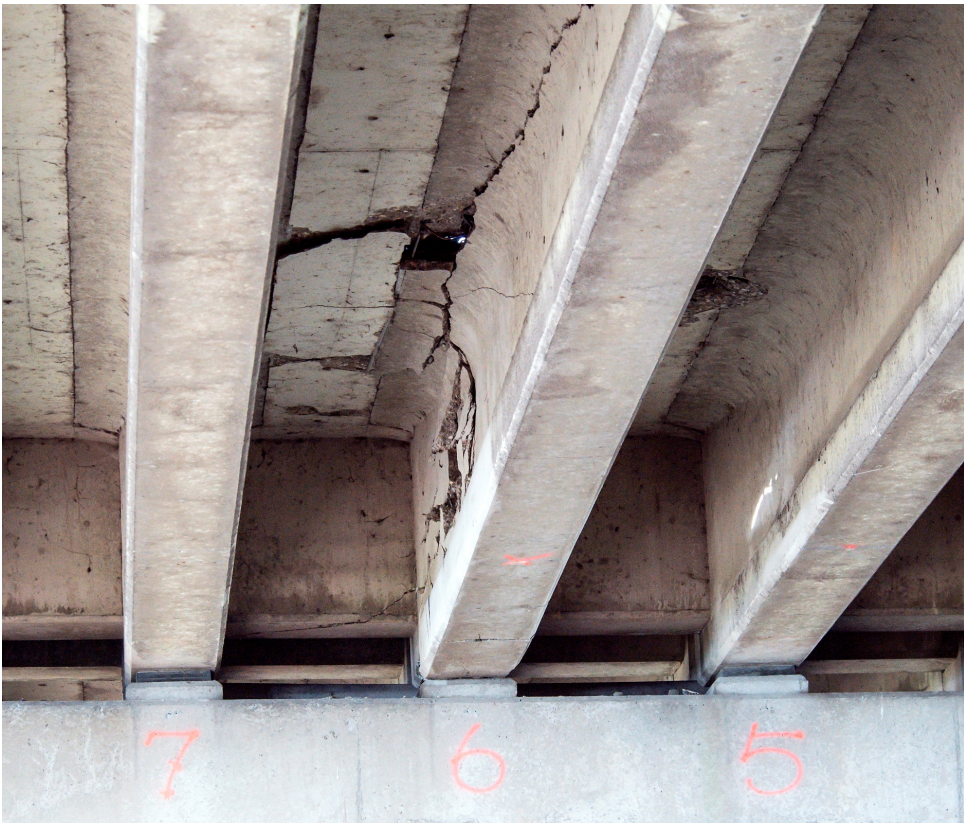
Figure 6.35: Punching failure deck slab and shear failure T-beam test 2, torsion crack end cross-beam (between T-beam 6 and 7)
