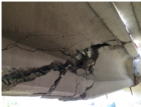
(a) Detail of shear crack (view towards span)
