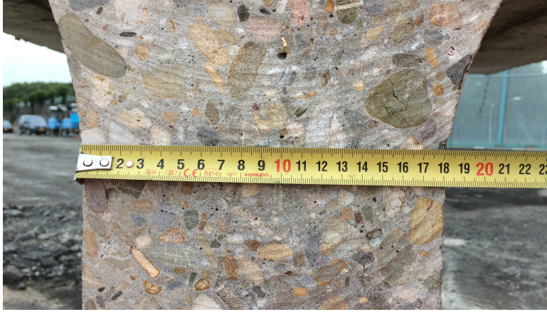
Figure 5.9: Saw cut of T-beam (web) showing large aggregates (measurements in cm)
