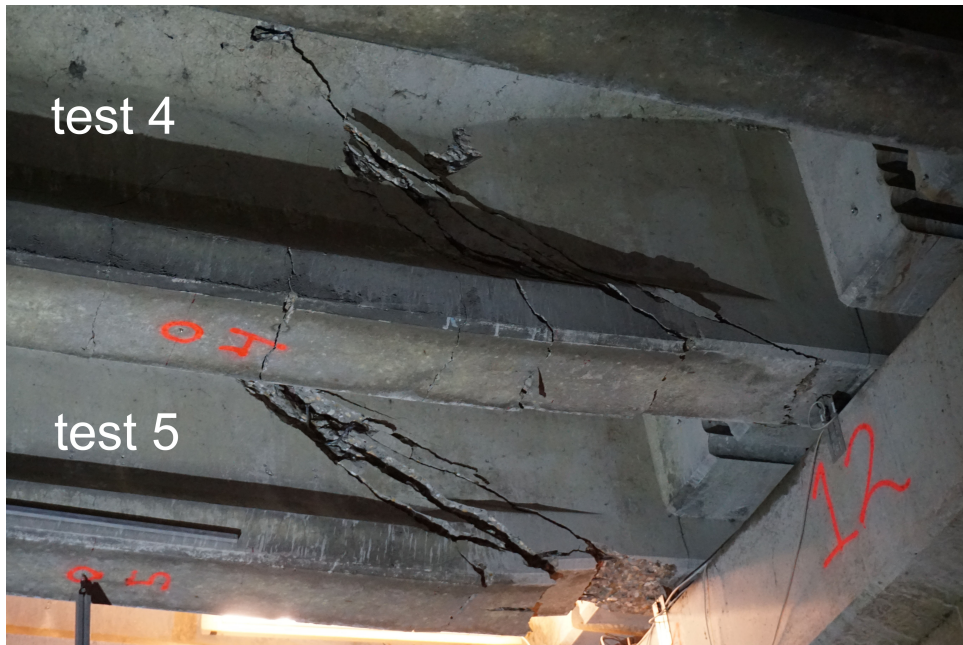
Figure 6.39: Flexural shear failure T-beam test 4 (top) and test 5 (bottom)
