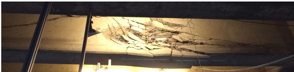
Figure 6.29: Shear failure T-beam test 1 (intermediate cross-beam on the left side, end support on the right side)
