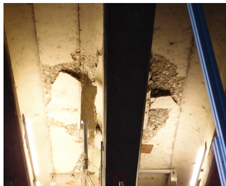
(b) Punching failure bottom side
