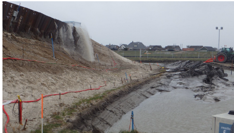
Figure 4.19: Failure of the dike (test site)
