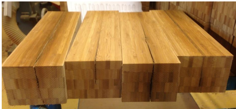
Figure 51 - Observed cracks in the glue lines
