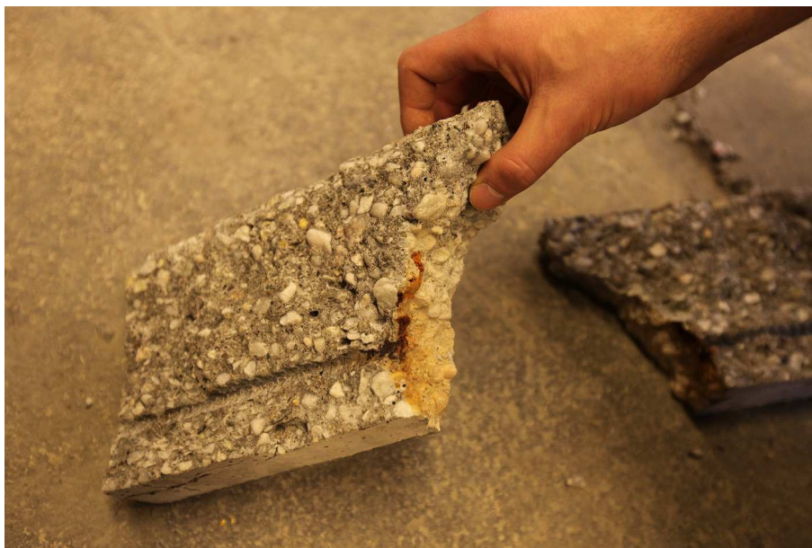
Figure 6 – Picture of the corroded cross-section after splitting (a part of) the beam
