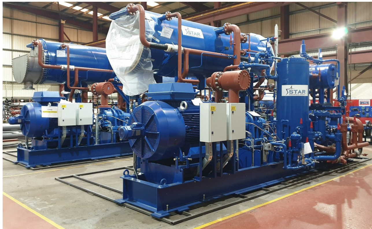
twin river source heat pumps at Queen's Quay, Clydebank, Scotland
