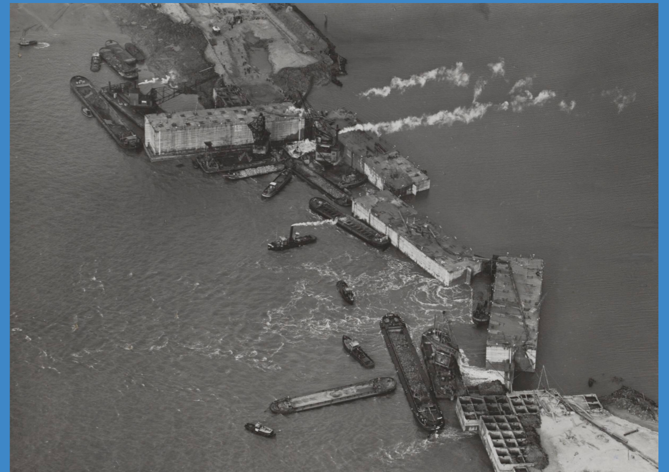
Figure 4.3: Aerial photograph of the closure of the breach at Ouwerkerk using Phoenix caissons (1953)
