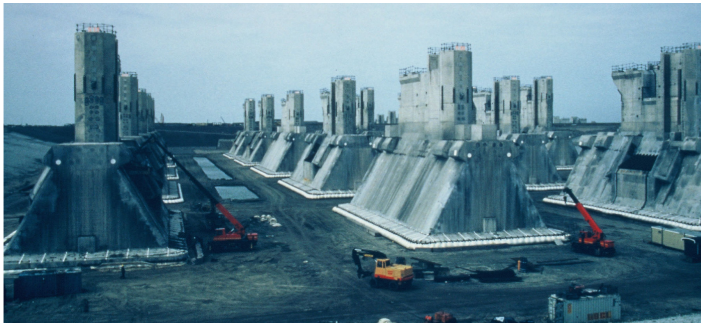
Figure 2.10: Each foundation caisson needed almost 7000m 3 of concrete. Between 1979 and 1983, 450.000m 3 of concrete was processed in the dock.
