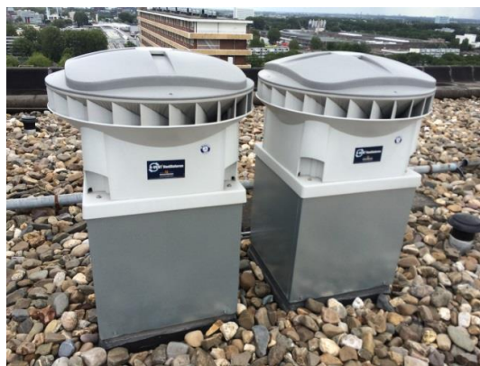
Figure 16: The ventilation exhaust on the roof
