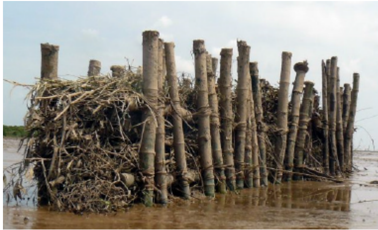
Figure 2.6: Example of brushwood groyne
