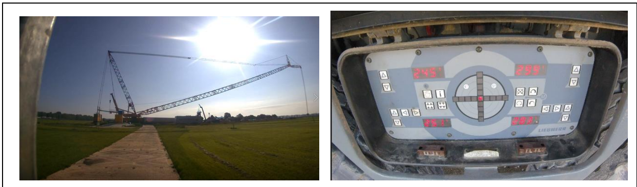
Figure 2: Pictures of the crane position as well as the outrigger pressures corresponding to measuring moment 15 of the boom rigging of WT4
