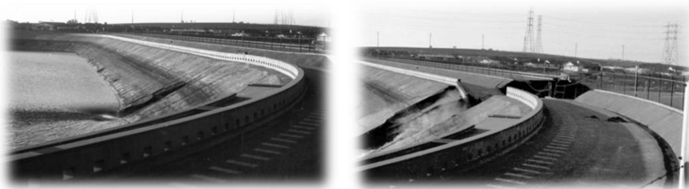
Figure 23: Initial crack formed in the embankment (on the left) and the development of the crack until collapse (on the right) (DHS and FEMA, 2002)
