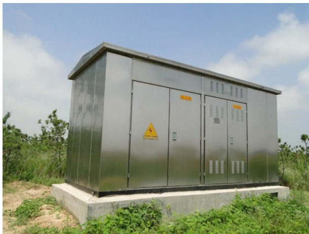
Figure 4-14: Impression electric substation (Smest, 2016)
