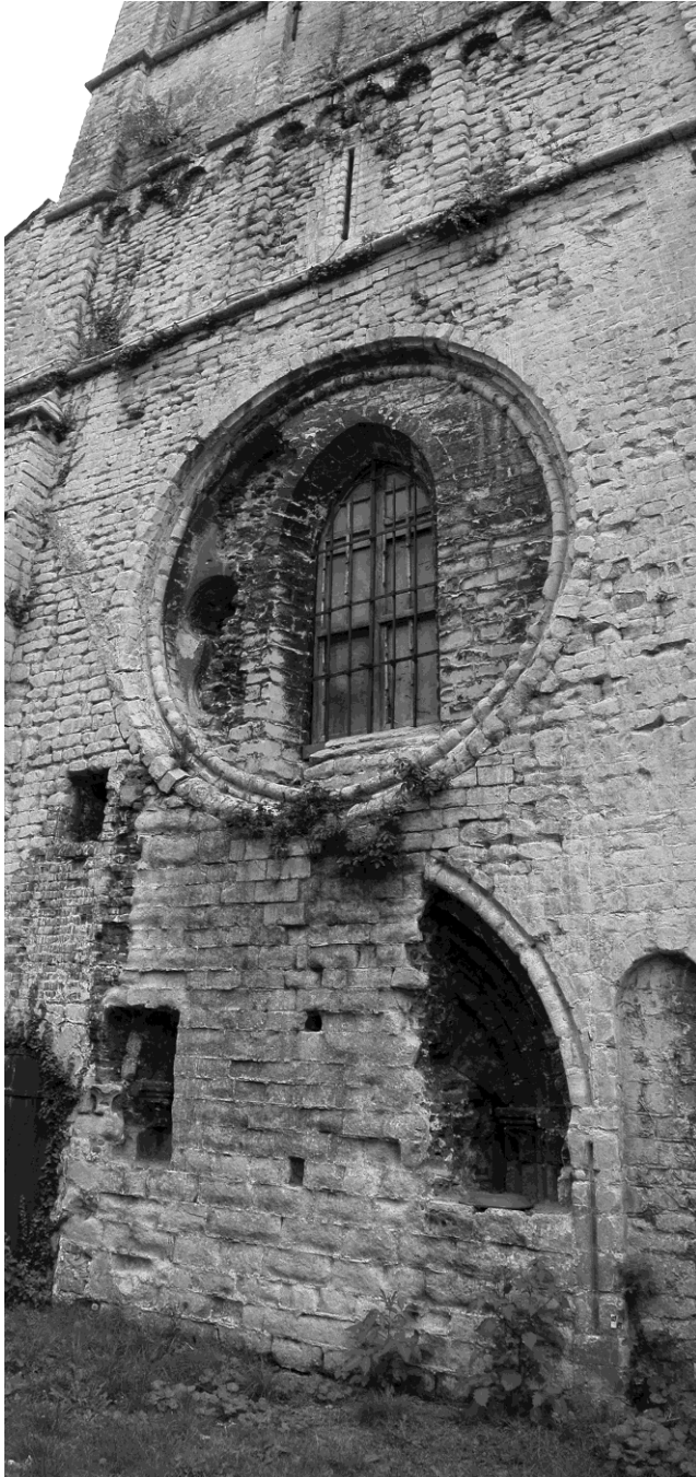
Figure 4.4: The original entrance to the tower of the church of Sint Jacob in Leuven (Belgium) now lies almost two metres below ground level.
