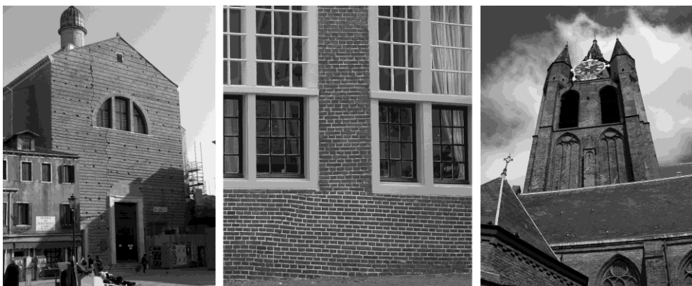
Figure 5.1: Three cases in which assumed structural damage is not damage. From left to right: church in Venice, Italy, where a joint resulting from an intervention may be misinterpreted as a crack (photograph by R.P.J. van Hees); so-called varkens to correct subsidence in houses next to the Hooglandse Kerk in Leiden; and kink in the tower of the Oude Kerk in Delft.
