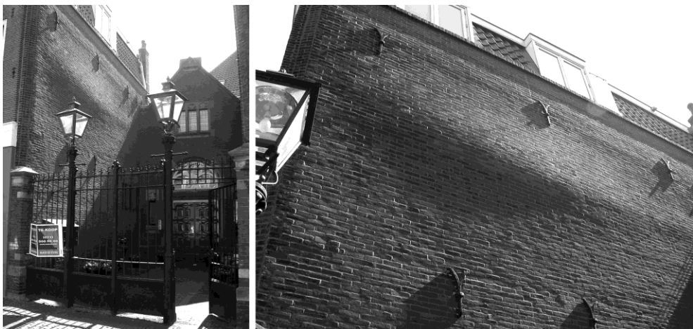
Figure 5.3: Deformation out-of-plane revealed by oblique lighting.
