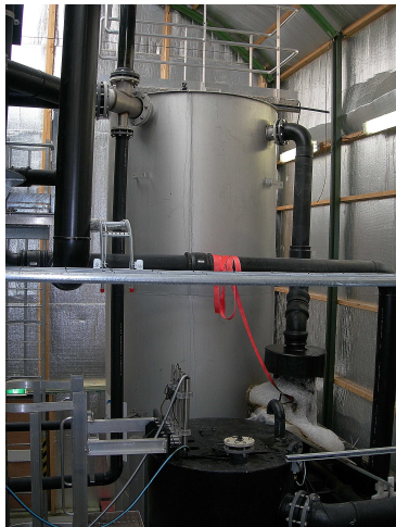
Figure 3-11 – Photograph of the continuous sand filter A at the Leiden Zuidwest WWTP
