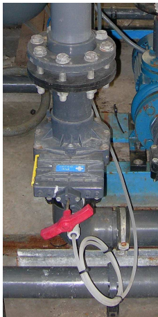
Figure 3-7 – Photograph of the initial mixing with a gate valve at the Horstermeer WWTP
