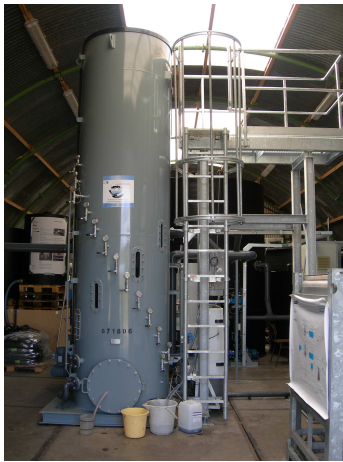
Figure 3-5 - Photograph of the 1-STEP ® filter at the Horstermeer WWTP
