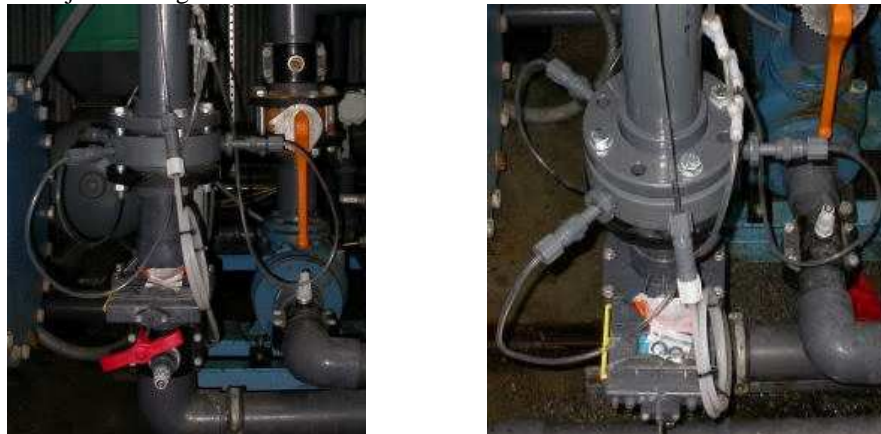
Figure 3-8 – Photograph of the initial mixing with an injection ring at the Horstermeer WWTP
