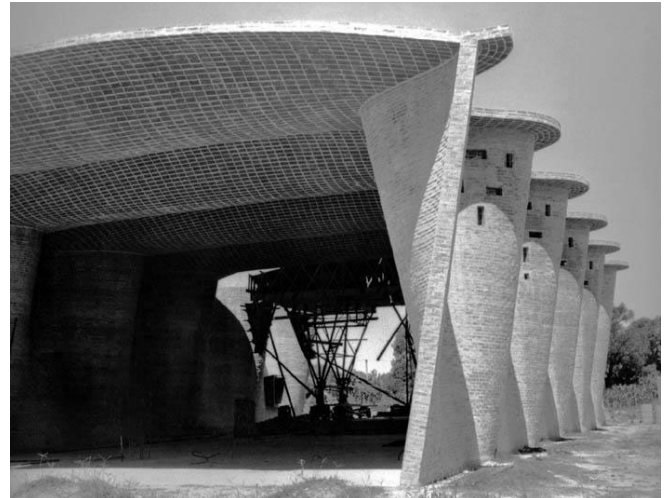
(b) - 'Church of Christ the Worker', Atlántida (close to Montevideo), Uruguay. This is a photo during construction. It was completed in 1960.
