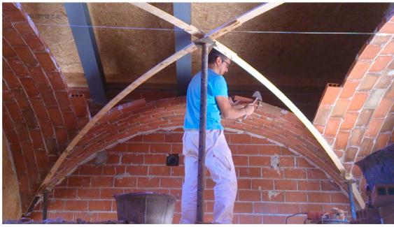
Fig. 1. Standard construction of a thin-tile vault in contemporary Spain using physical guidework — by Salvador Gomis Aviño.
