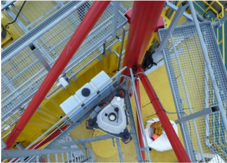
Figure 4.3: Top view of LiDAR installation at IJmuiden
