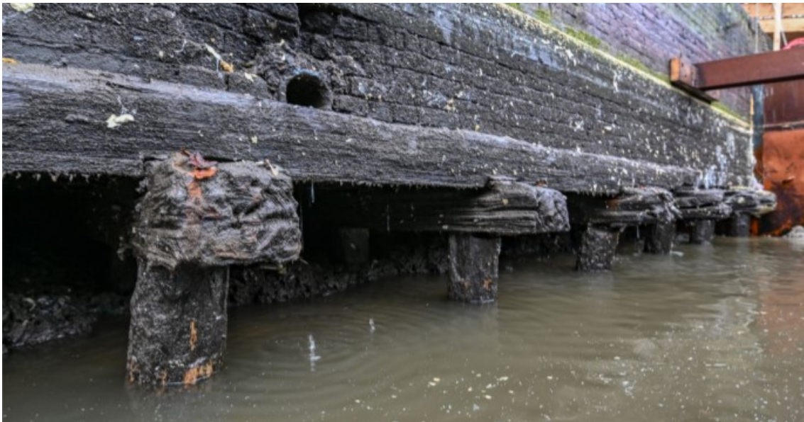
Figure 2.6: Wooden foundation structure from an old quay wall undergoing renovation (taken at Da Costakade, december 2018), retrieved from the municipality of Amsterdam.
