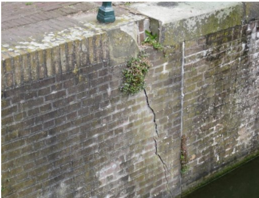
Figure 2.8: Damaged quay wall near a dilation joint, retrieved from (de Gijt et al., 2013).
