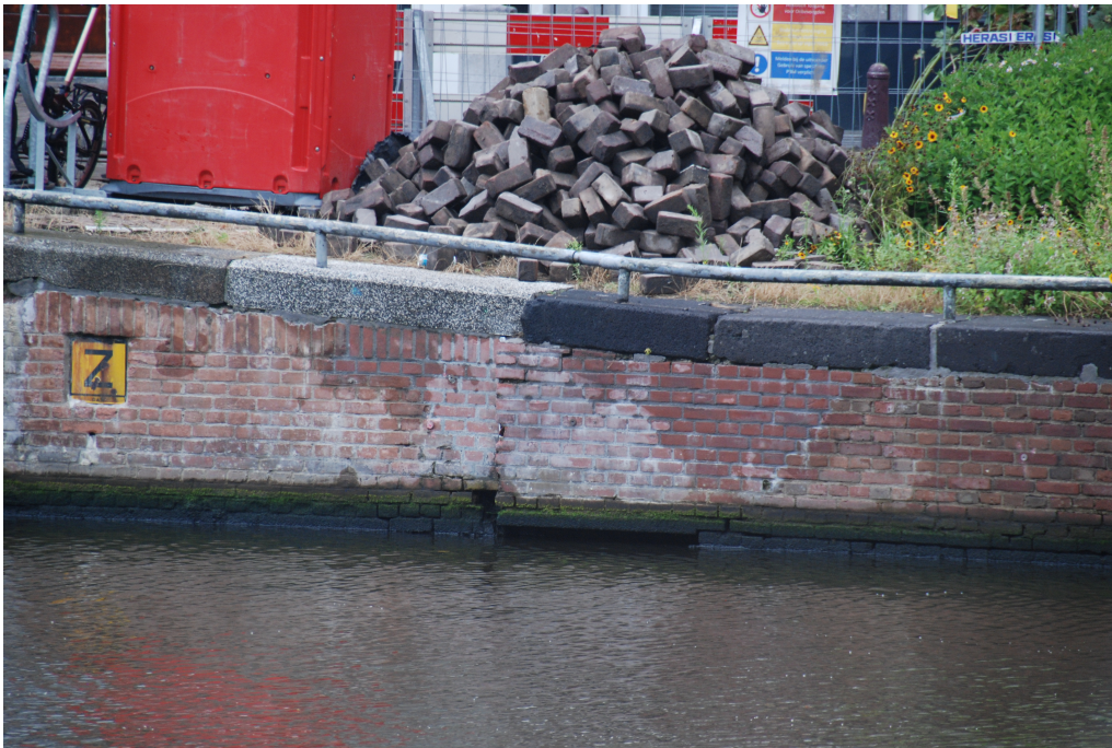
Figure D.7: Sixth photo of the quay wall at "Nieuwe Herengracht". Shows the other side of the quay wall with damaged bricks and what appears to be a relatively thin diagonal crack moving up to the right, at the right-hand side of the dilation joint.
