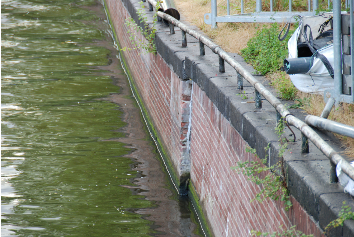
Figure 6.4: Photo of the quay wall at "Nieuwe Herengracht". Quay shows movement towards the water as the masonry sticks out at the dilation joint.
