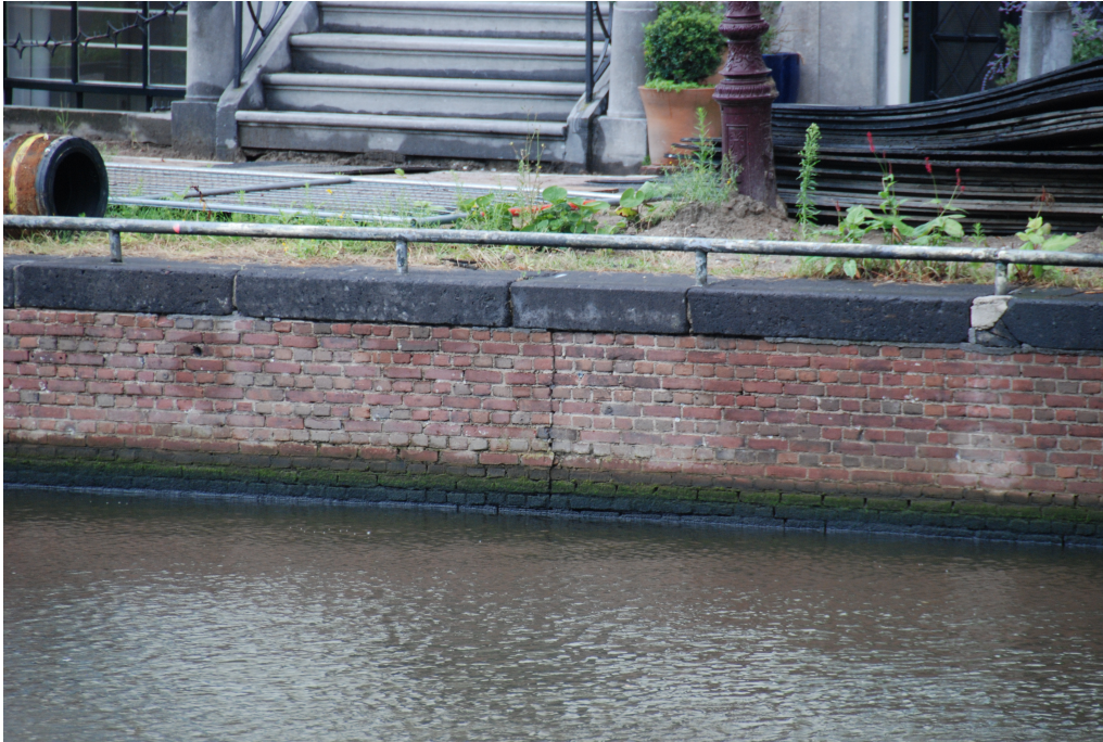
Figure D.6: Fifth photo of the quay wall at "Nieuwe Herengracht". Relatively uniform vertical crack along with relatively small gaps between individual bricks at the lower side.
