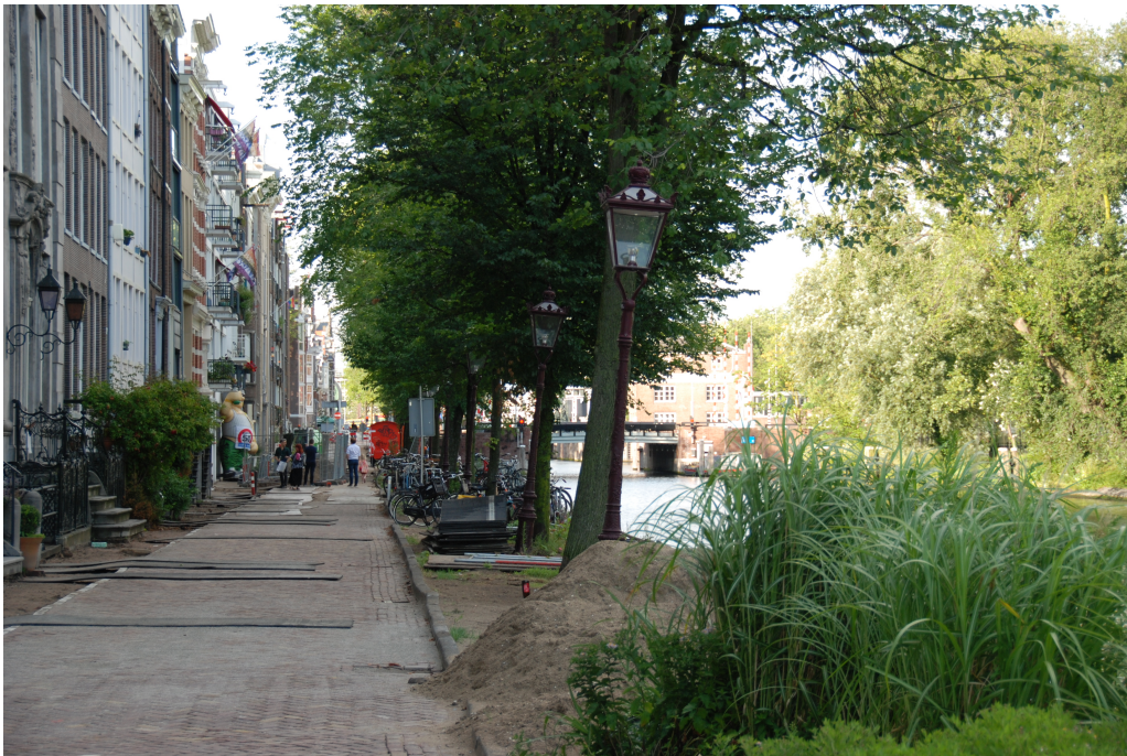
Figure D.9: Side view of the quay wall at "Nieuwe Herengracht". Street lanterns all tilt towards the water, indicating a forward tilt of the entire structure.
