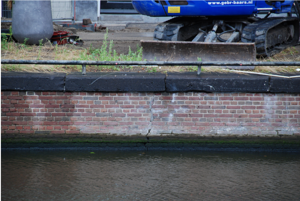
Figure D.4: Third photo of the quay wall at "Nieuwe Herengracht". Vertical crack along with gaps between individual bricks at the lower side.
