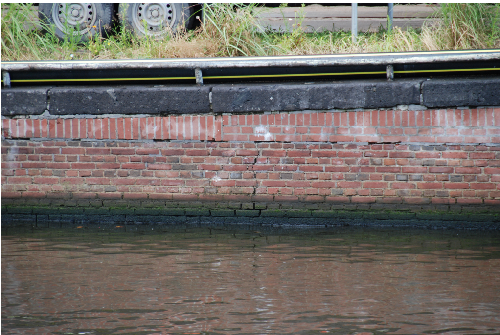
Figure D.3: Second photo of the quay wall at "Nieuwe Herengracht". Vertical crack along with gaps between individual bricks at the lower side.
