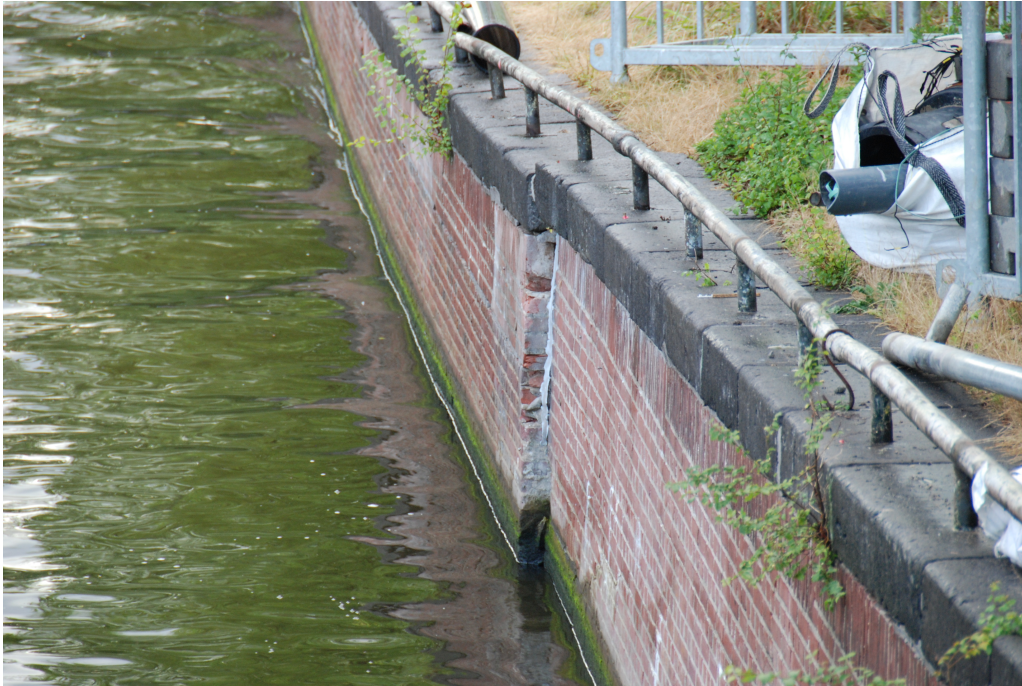
Figure D.2: First photo of the quay wall at "Nieuwe Herengracht". Quay shows movement towards the water as the masonry sticks out at the dilation joint.
