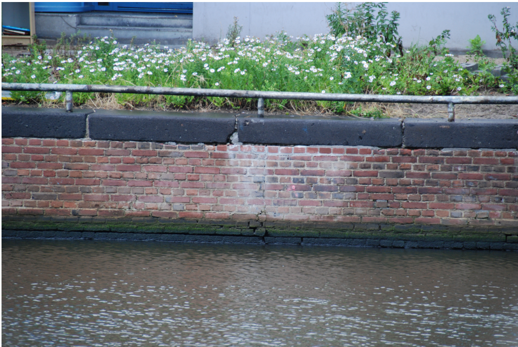
Figure D.5: Fourth photo of the quay wall at "Nieuwe Herengracht". Vertical crack along with gaps between individual bricks at the lower side.
