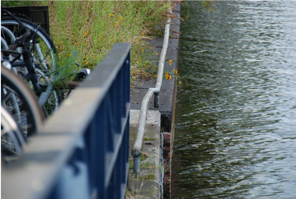
Figure D.8: Sixth photo of the quay wall at "Nieuwe Herengracht". Quay shows movement towards the water as the masonry sticks out at the dilation joint at the Southern end.
