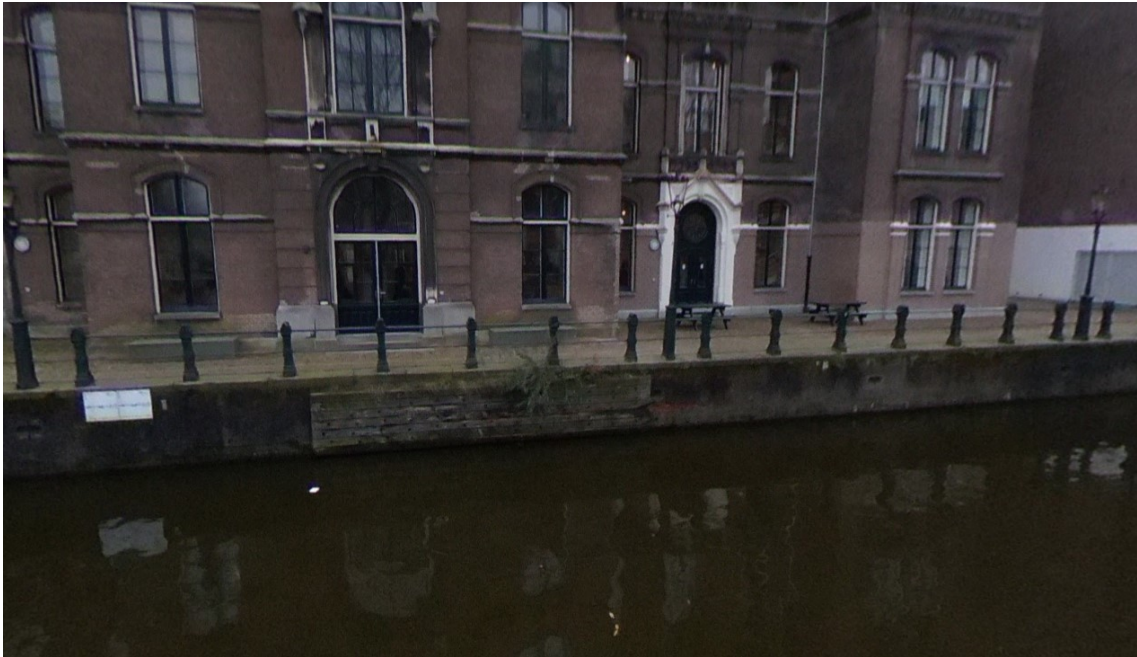
Figure 1.1: Grimburgwal before collapse (Amsterdam) in feb. 2018 (Google Street View).
