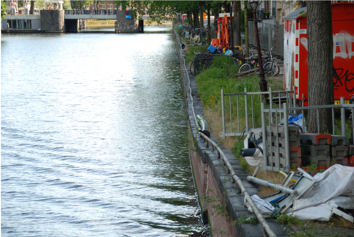
Figure D.10: Side view of the quay wall at "Nieuwe Herengracht". Masonry wall shows general forward tilting.
