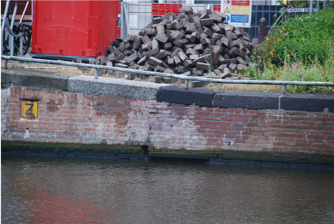
Figure 6.7: Photo of the quay wall at "Nieuwe Herengracht". Shows the other side of the quay wall with damaged bricks and what appears to be a relatively thin diagonal crack moving up to the right, at the right-hand side of the dilation joint.
