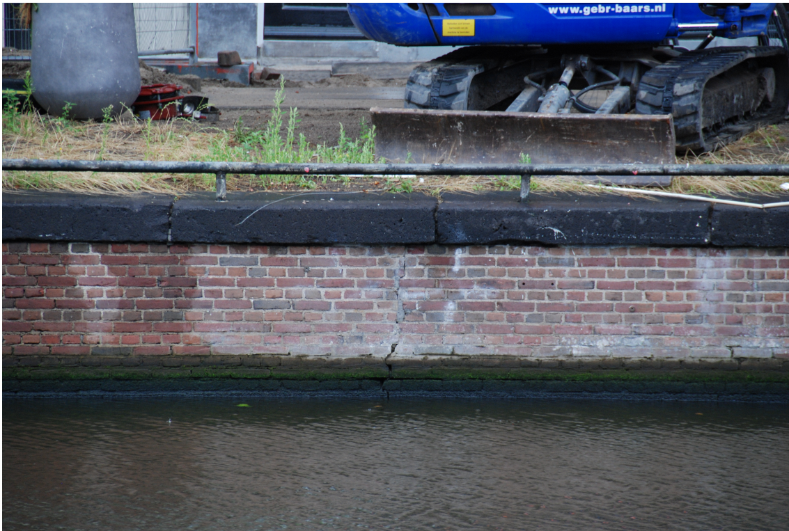
Figure 6.6: Photo of the quay wall at "Nieuwe Herengracht". Vertical crack along with gaps between individual bricks at the lower side.
